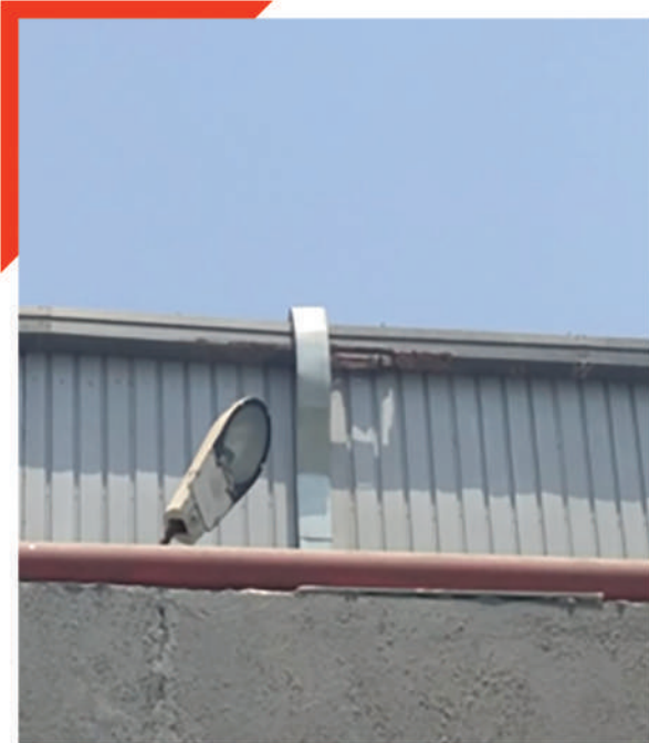
Damaged Gutter (Before)
